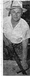
HARD-WORKING Baptist minister, the Rev. Richard Walker, 49, sawing timber yesterday to put the finishing touches to his new manse in Alexander Street, Clayfield.
